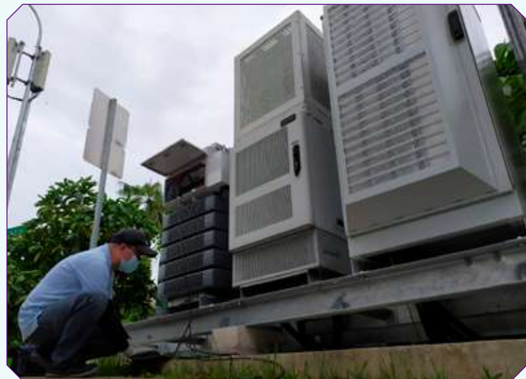
StarHub's mobile base stations across Singapore are used as rainfall sensors.
