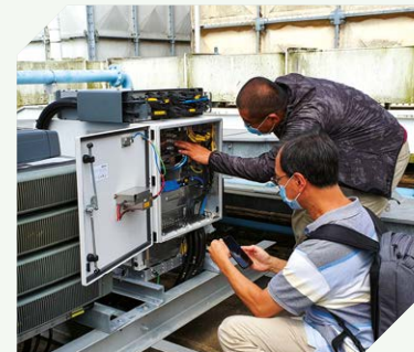
Engineers checking the signal strength of a mobile base station.
