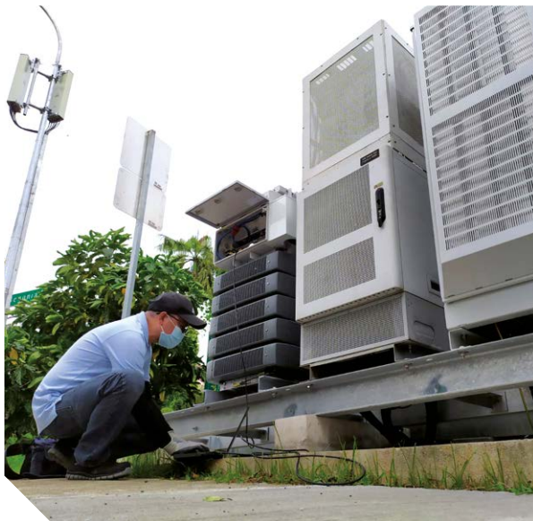
Engineer maintaining a mobile base station.
